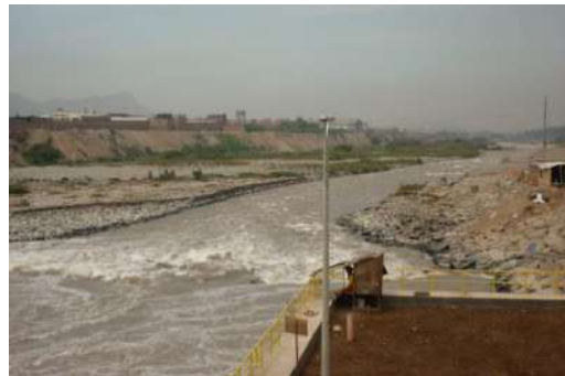
Figure 2. Incision in the right bank in the bed downstream of the stilling basin in Huachipa Diversion Dam
