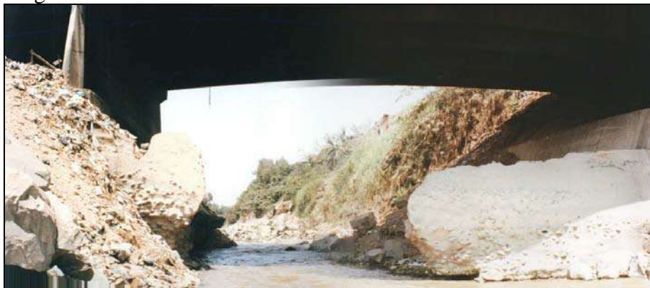
Figure 4. Scour under the Duenas Bridge. Notice the grade control structure built in 1977 that was completely destroyed in 2001.
